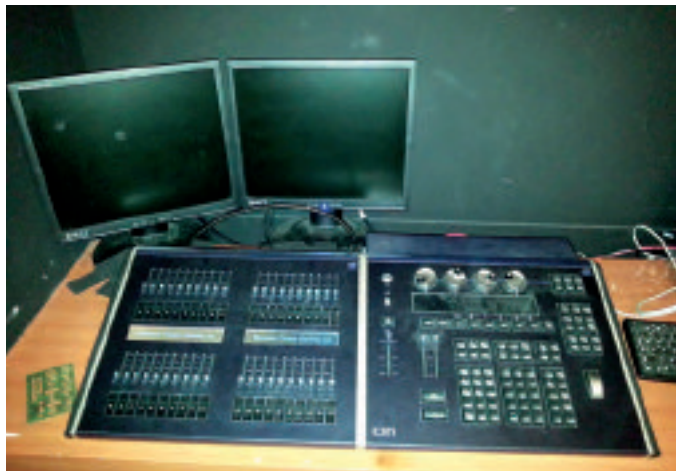
Lighting consoles can control a variety of devices beyond the standard dimmer and conventional fixture
